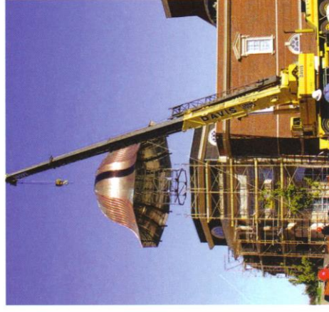
Parkway Hills Baptist Church, Plano, Texas, phase 3 of construction; Rogers-O'Brien Construction Company, contractor; Leo A. Daly, architect
